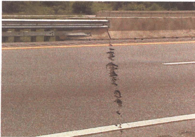
POTHOLE @ JOINT B-APPR-TYPICAL
